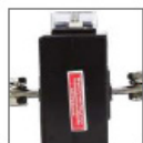
The transformer housing is not intended to be open and is additionally protected by an anti-tamper sticker to prevent access to the secondary winding.
